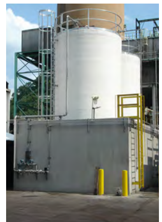
CORMETECH's design urea unloading and storage facility
